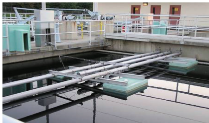
Maroochy Shire sewage plant (2000)
